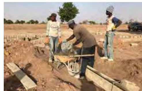
Workers excavating the ground and laying the foundation and the exterior walls.
